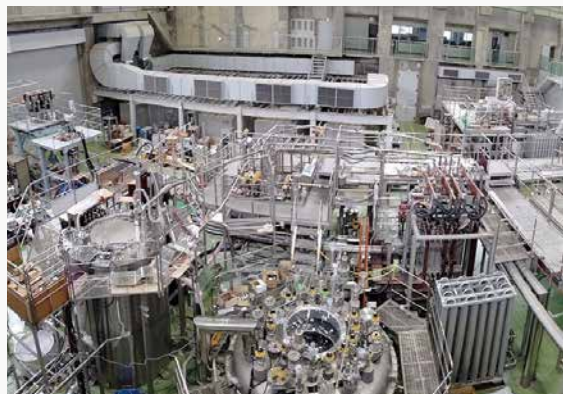
Superconducting conductor test facilities in Superconducting Magnet System Laboratory
